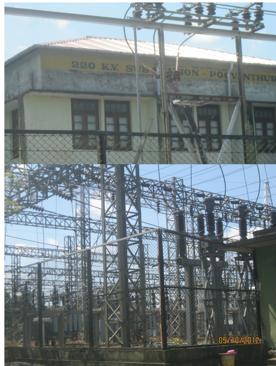
220KV Poovanthuruth substation
